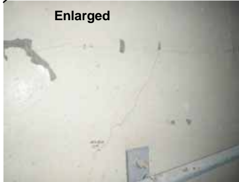
2. Inner surface of the second floor west exterior wall between W3 and W4 (Crack width: 0.3mm)
