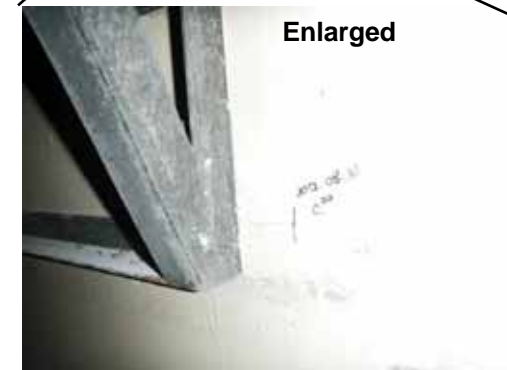
3. Inner surface of the second floor west exterior wall between W4 and W5 (Crack width: 0.2mm)
