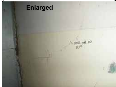
1. Inner surface of the second floor west exterior wall between W2 and W3 (Crack width: 0.1mm)
